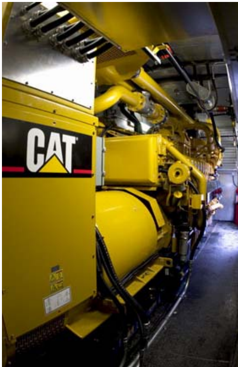
PHOTO 1 LANDFILL GAS GENERATOR SET AT THE HARTLAND LANDFILL IN VICTORIA, BRITISH COLUMBIA
