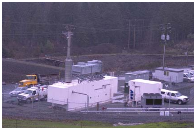
PHOTO 2 POWER GENERATION STATION AT THE HARTLAND LANDFILL SITE
